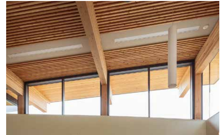
Clerestoreys reduces need for the LED integrated lighting..
