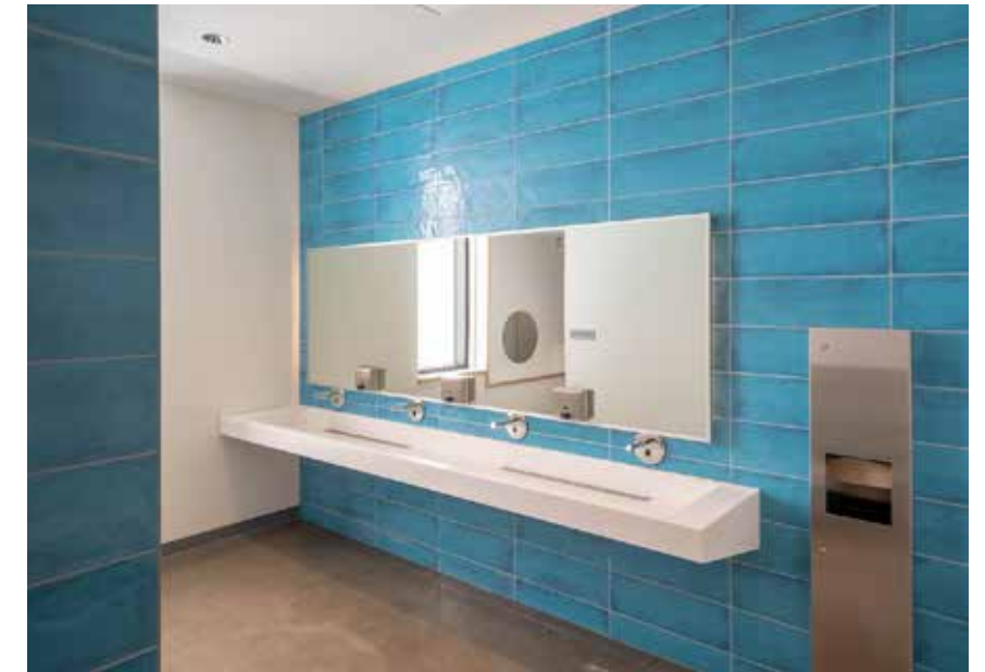
Daylit washrooms feature low flush fixtures and a communal sink area for inclusion and equality.
